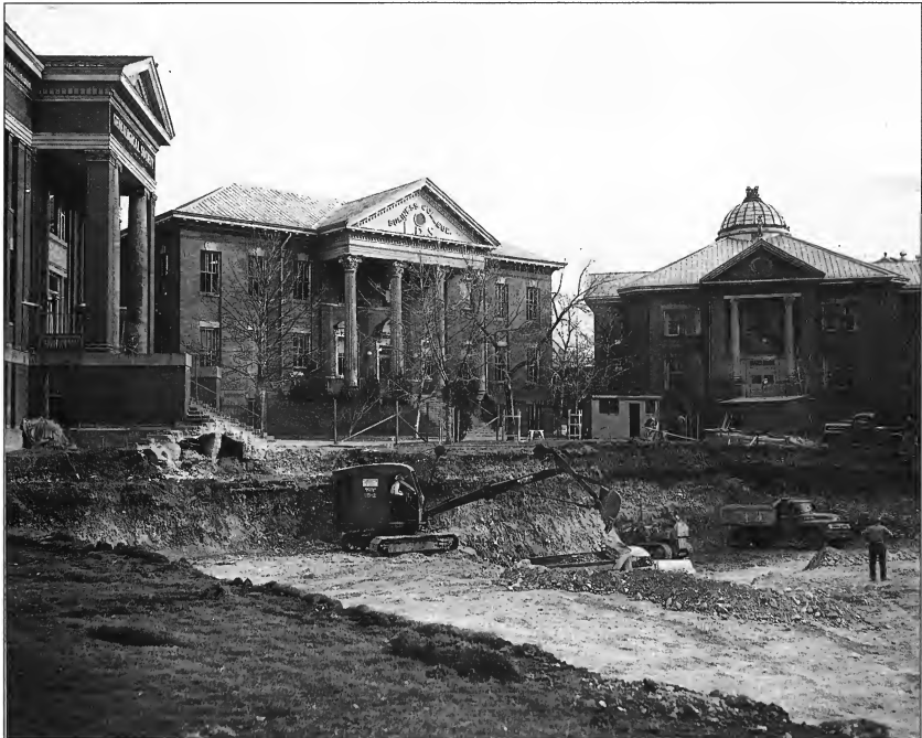
DEMOLITION OF THE OLD LDS UNIVERSITY, LDS BUSINESS COLLEGE CAMPUS AT 70 NORTH MAIN STREET IN 1961 TO MAKE WAY FOR THE 26-STORY CHURCH OFFICE BUILDING.
